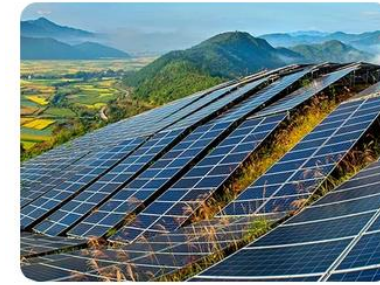
Support structure components
